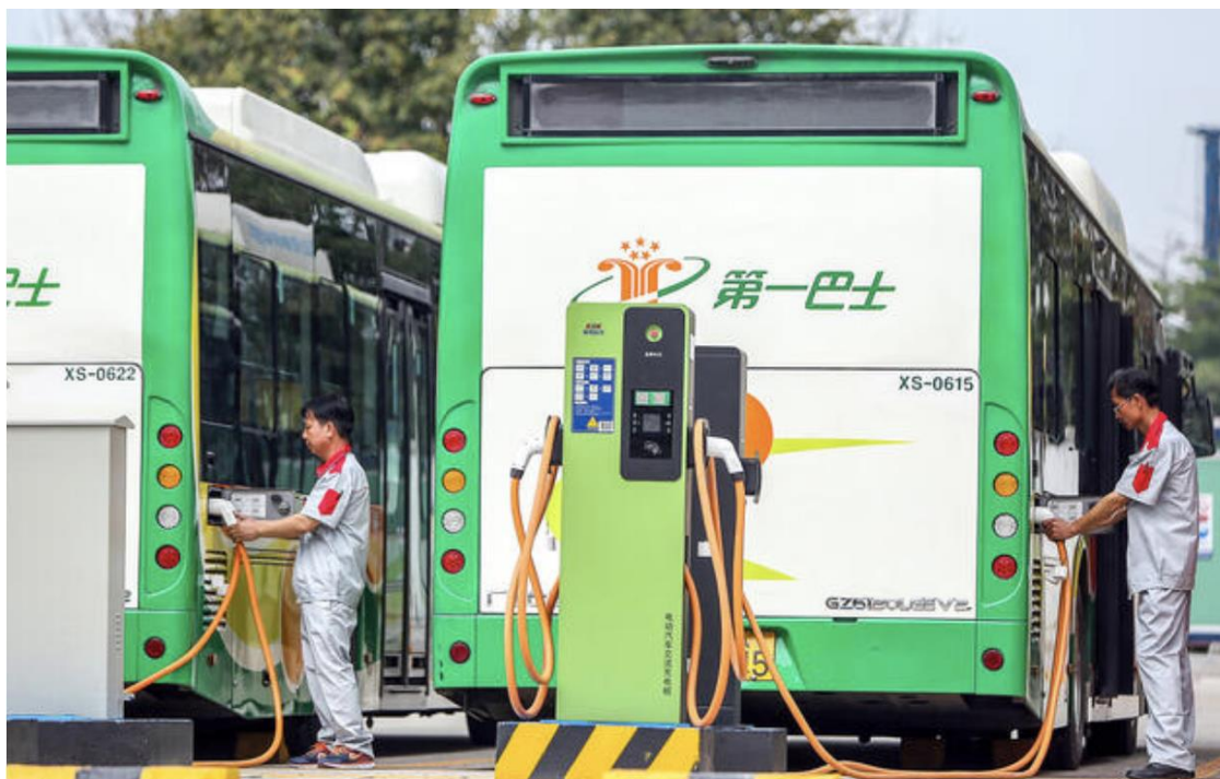
Figure 2. Charging infrastructure in Guangzhou City, China
